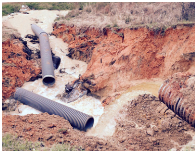
In March 2016, floodwaters dug a 50-foot wide hole on the downstream end of this dam. Delos Dewayne Collins/Texas Observer
